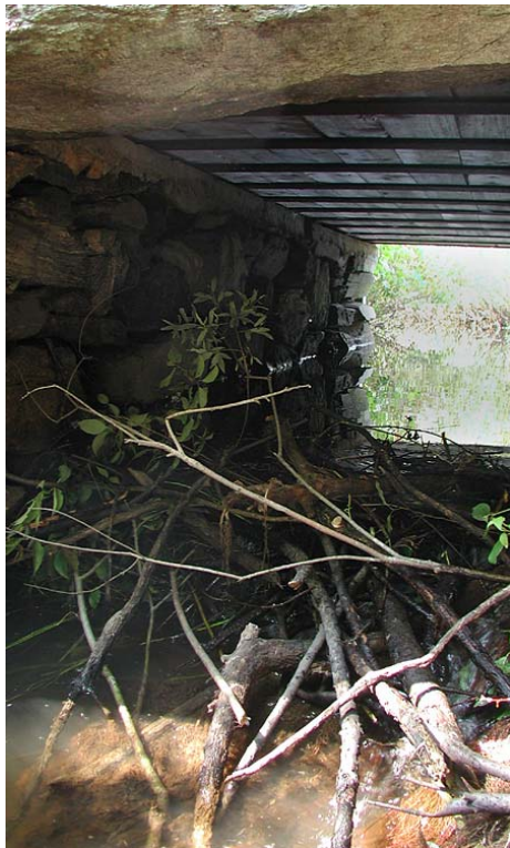
Figure 12: Beaver dam blocking road culvert, Cold Harbor Brook, Sept 2005
